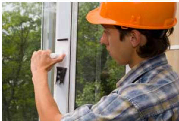
Putting up storm windows in autumn and remove them in spring to reduce winter heat loss by up to 50 percent.
